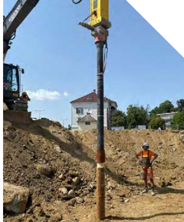
SECOND TRIAL: COMBINATION OF TIMBER PILE with ductile pile attachment in the area of changing groundwater levels
